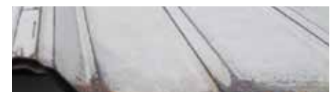
Advanced stages of rust and paint deterioration on each bend of a cold-formed panel.
